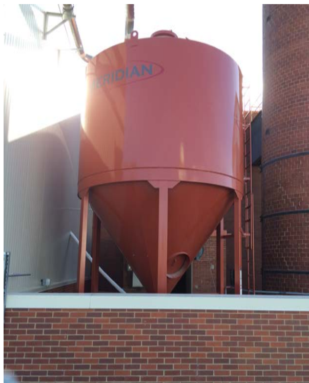
Figure 2.2: Primary Fuel bin
